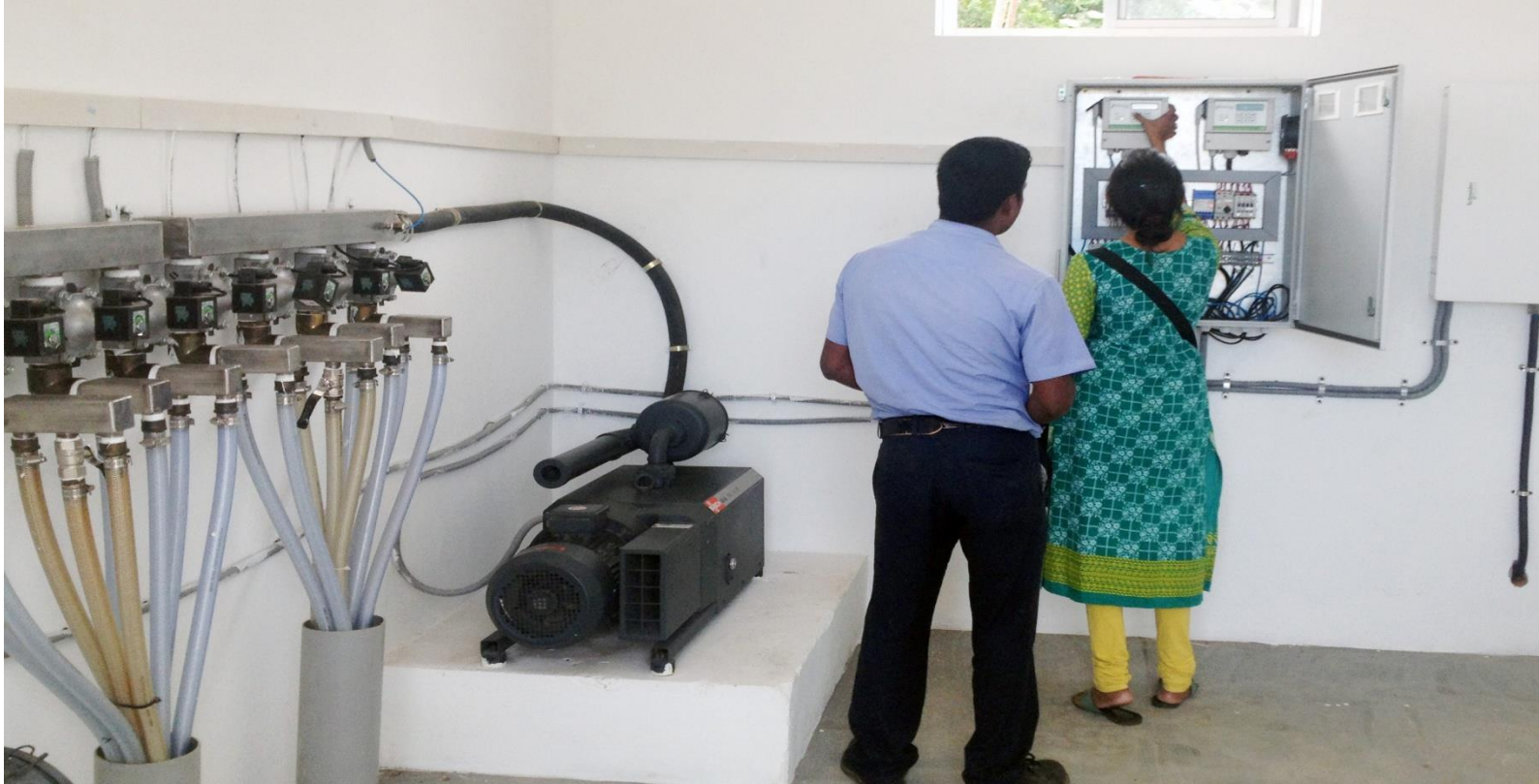
130 KLD EcoSBR plant in an educational institute-Chennai
